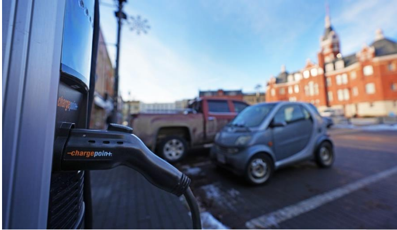
Figure 9 Electric charging station at Market Square
