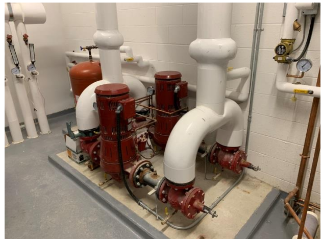
Figure 3: Dual Pump Geothermal Exchange System
